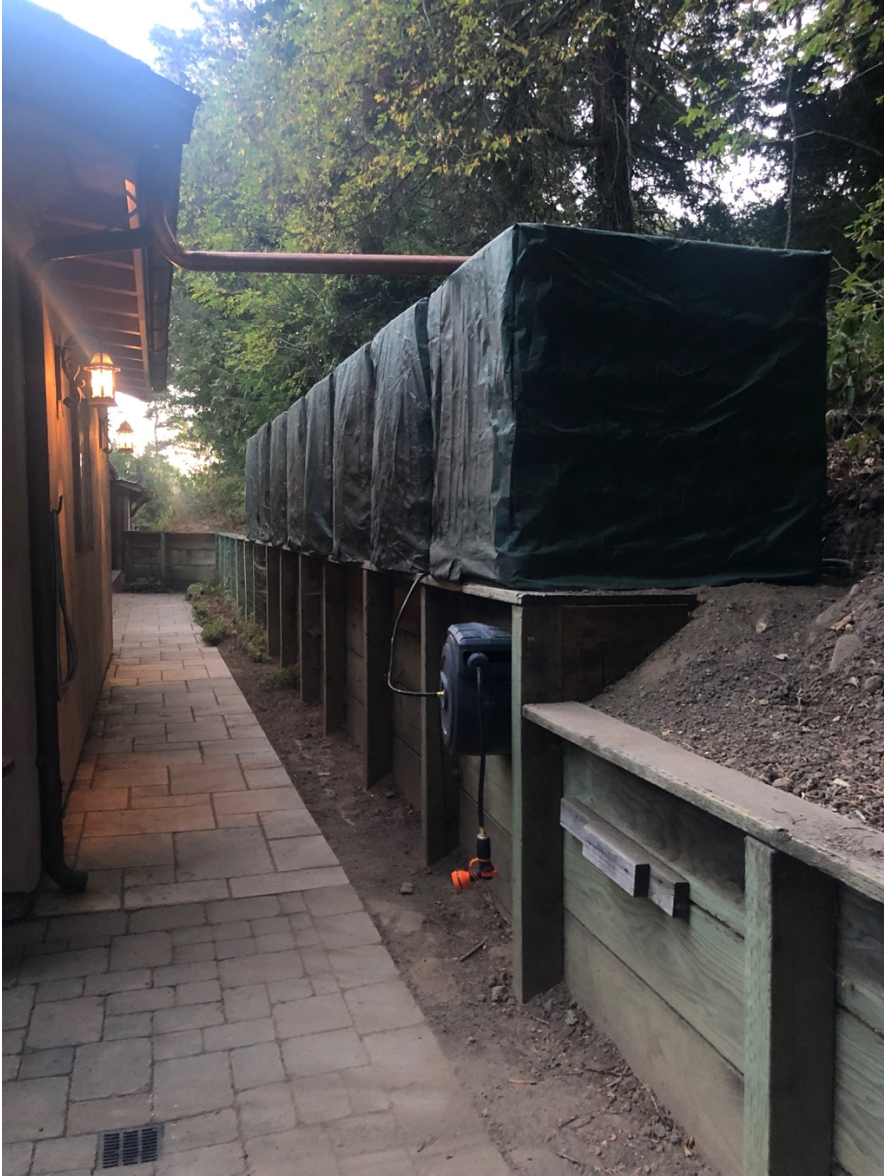
Upper Tank Bank
